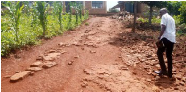
The road to the school was not accessible
