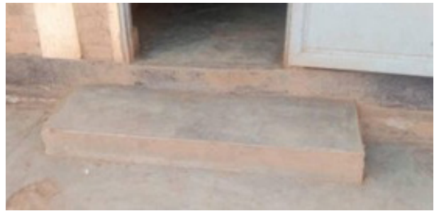
Steps were a significant access issue for many classrooms
